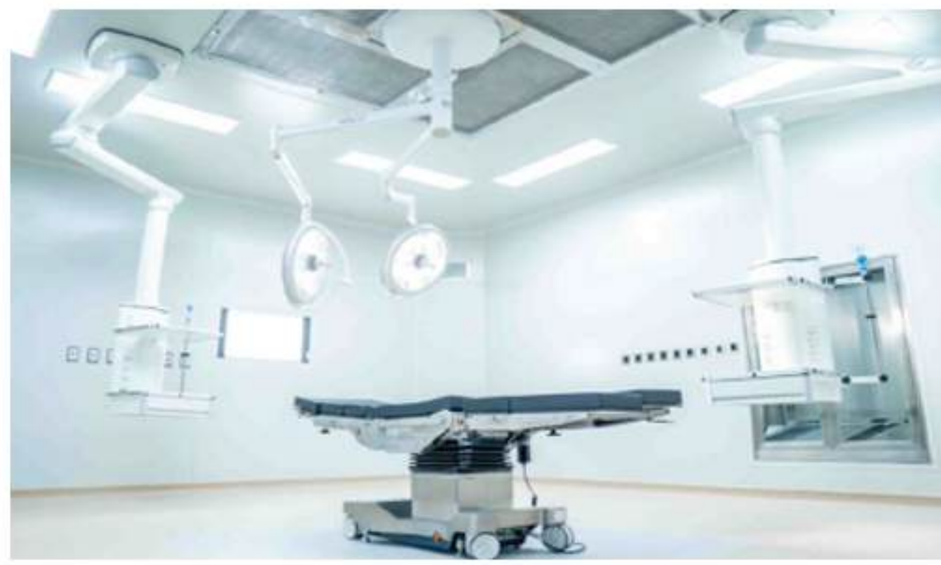
MODULAR OPERATING THEATRE
